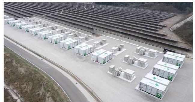
Panoramic view of storage battery facilities
